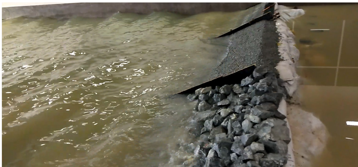
Figure 5 Wave run-up on different revetments at the same time (picture taken 25 November 2018).
