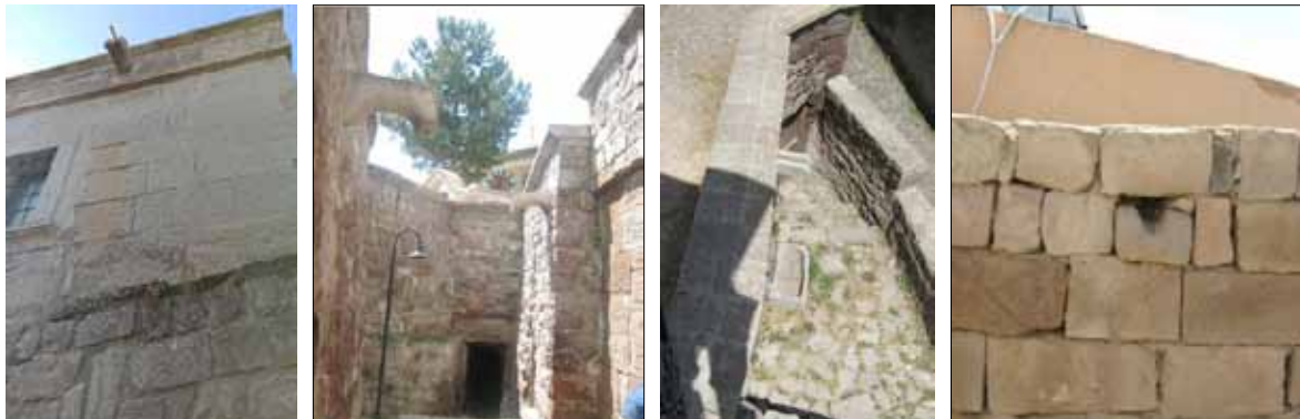
Figure 17. Left 2 pics, roof waterspouts and center right courtyard walls to drain rainwater. (Source: Photos by authors).
