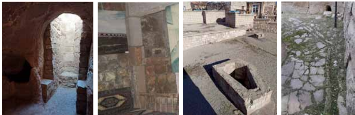
Figure 7. Left & 2nd from left, bathing areas. Third from left, lighting and ventilation shaft above the bathing area with its extension on the flat roof and (right) open gutters in the courtyard for surface drainage. (Source: Photos by authors).
