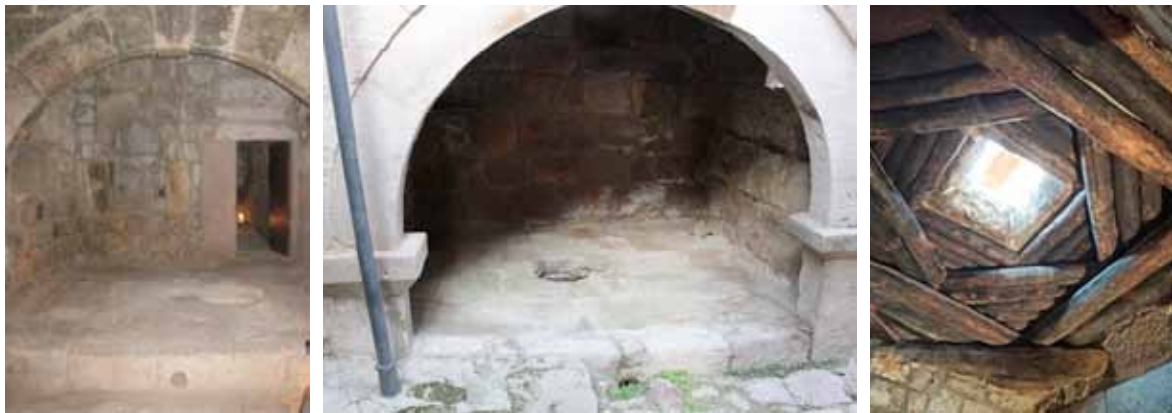
Figure 3. Tandoor pits (left & center) with their ash-discharge holes and stone sliding cover ( duvak ) & wooden lantern-roof/ tüteklikli örtü . (right) Above the tandoor room in the stone masonry section. (Source: Photos by author).
