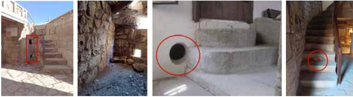
Figure 11. Ventilation holes on the walls and steps specially built for ventilation of cellar spaces. (Source: Photos by authors).
