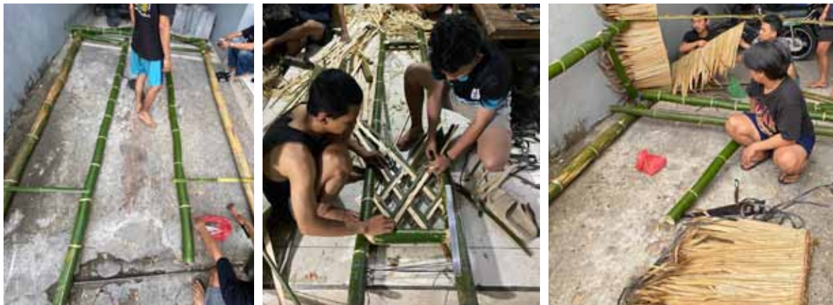
Figure 8. (Left) Making the structural posts of the Baruga, (Center) Weaving the Baruga walls, (Right) Installation of the Baruga roof use Nipa leaves.
