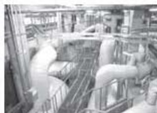
Centralized management of lifelines [Joint utility tunnels]
