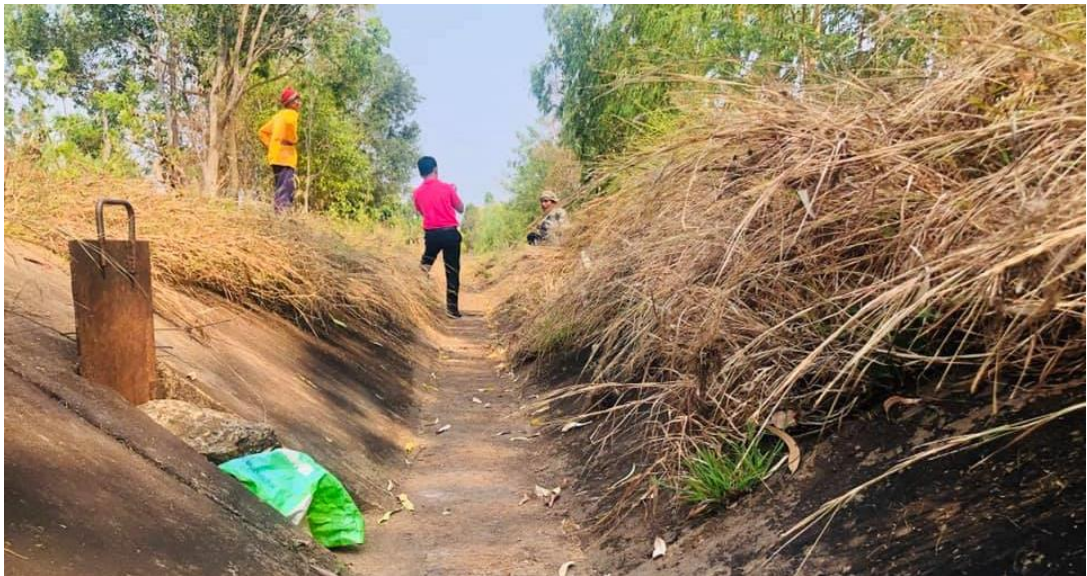
Figure 3. A Damaged Canal
